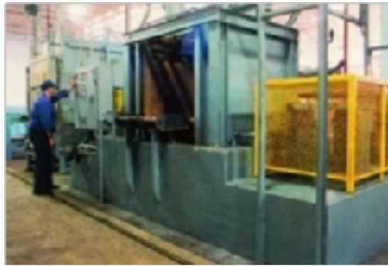
Figure 4 6,000-gallon IQ tank across the aisle from 36"x36"x48" atmosphere furnace installed at Akron Steel Treating Co.
